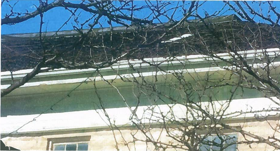
South facing roof. Curling is visible from train platform and Park Avenue.
