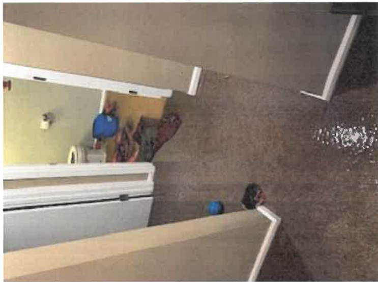
Bathroom hallway during flood
