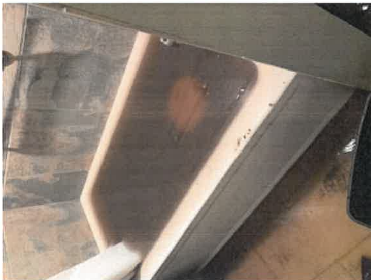
Bathroom 1 during flood
