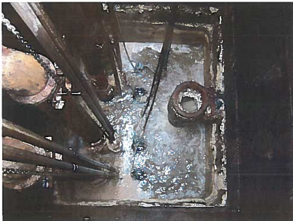
Yorktown Lift Station after cleaning
