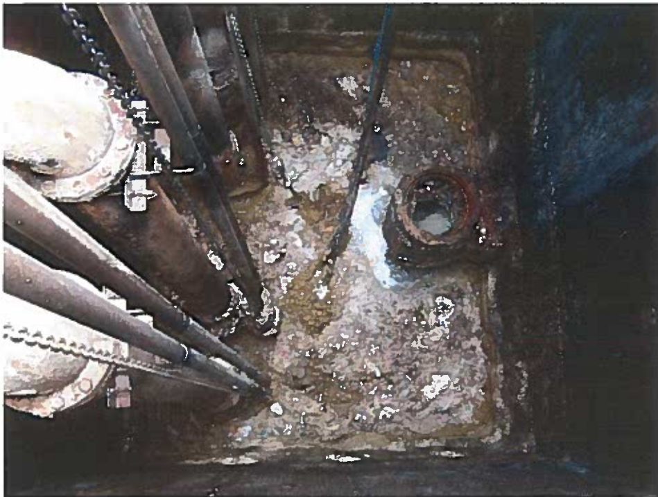
Grease build-up at Yorktown Lift Station
