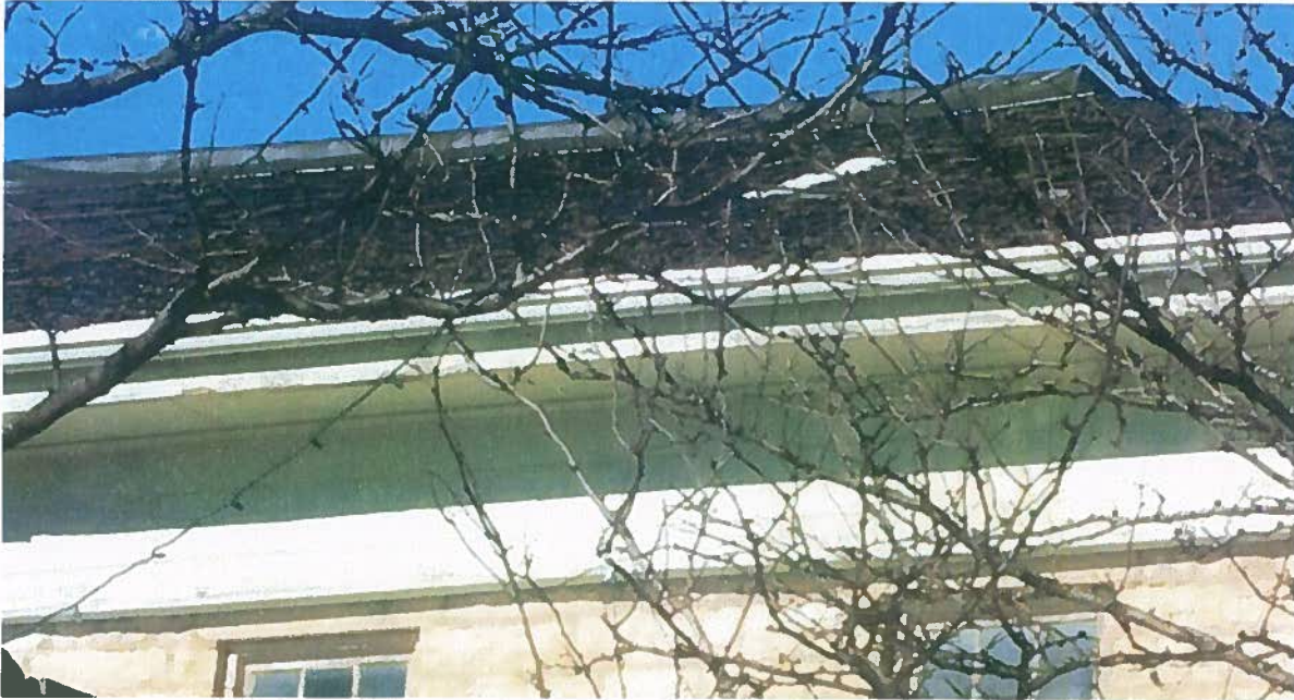
South facing roof. Curling is visible from train platform and Park Avenue.
