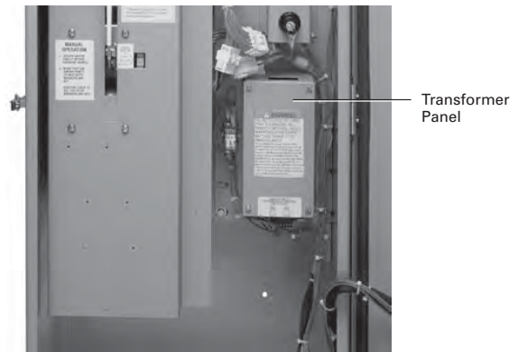
Transformer Panel Location
