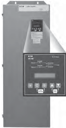
Wall-Mount Transfer Switch
