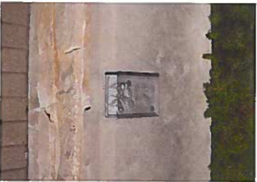
Starboard Deteriorated Metal Band
