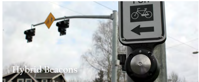
Route Users to Existing Signals
