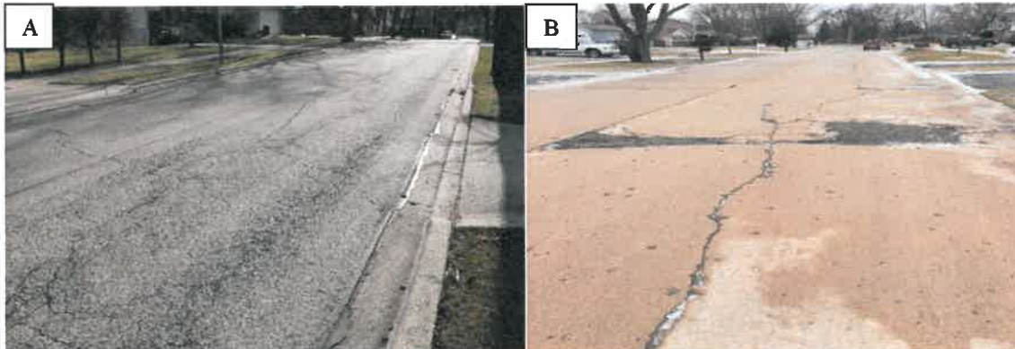
Figure 10: (a) Garfield Terr between Hickory St and Washington Blvd with a 40 PCI (b) Fairfield Ave between Pleasant Ln and Berkshire Ave with a 41 PCI
