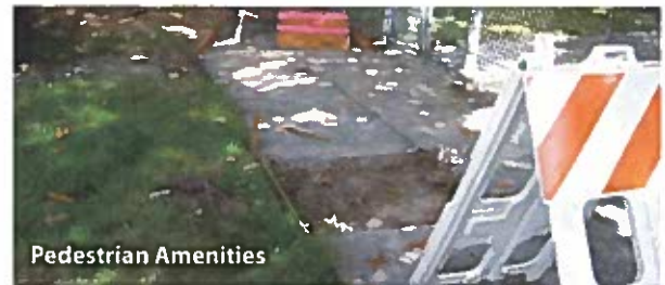
Sidewalk Obstructions and Driveway Ramps
